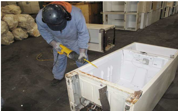
Jaco Environmental removing insulation foam Under contract to EOS Climate Photo Credit Christopher Joyce/NPR
